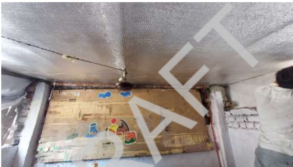
Figure 41: Alufoil Static (under a tin-roof)
